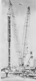
Fingering the sky here are the V-shaped boom end mast of the Manitowoc Crane setting one of the catacarb towers in place.
